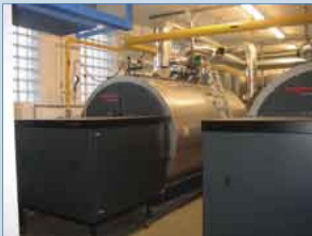
Technologie kotelny, Vimperk Boilers new situation, Vimperk
